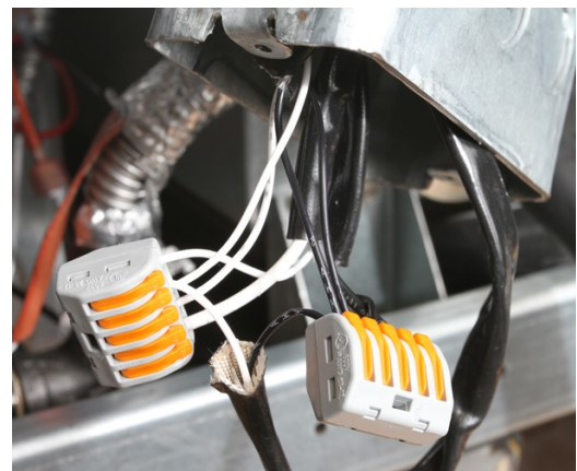
Fig 12 Wago connectors shown in junction box.
